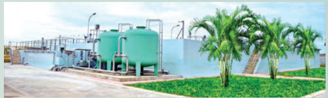
Bac Dong Phu Industrial Park consistently prioritizes wastewater treatment
