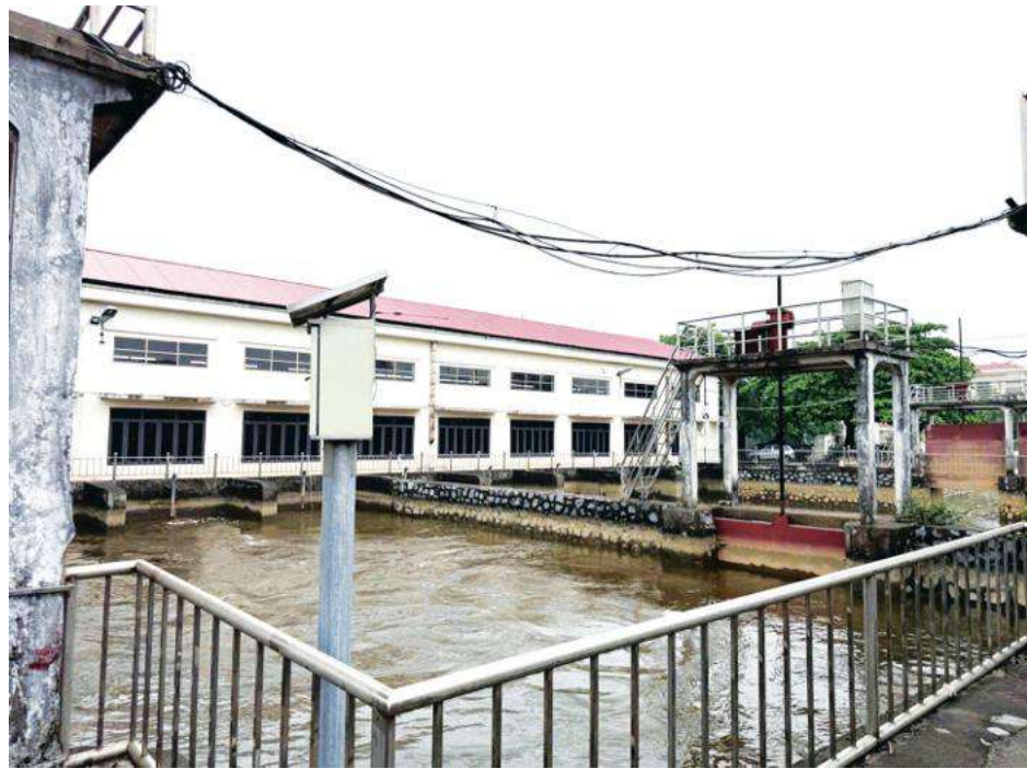
Automatic water level monitoring station
